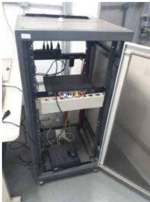
71. RACK COM SWITCH DELL 2724
