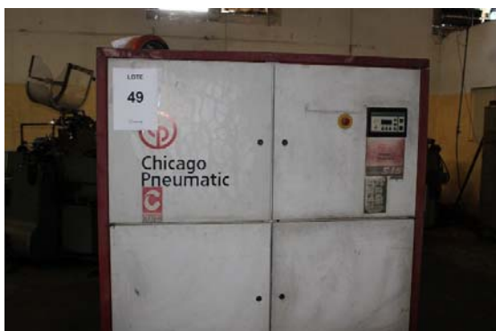
Lote 049 - Compressor Chicago Pneumatic S15-1
